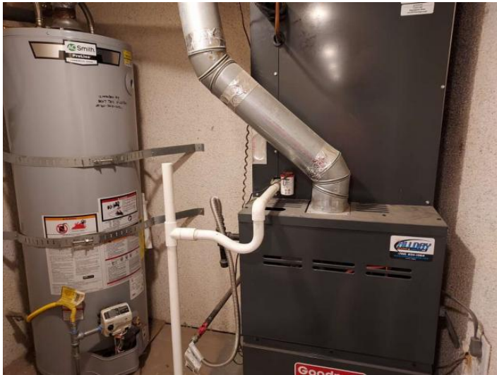
Mechanical Closet Hot Water Heater with Dual Earthquake Strapping
